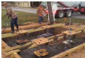
Foundation preparations for the 30-foot-tall Veterans Tribute Tower 2014-2015 at Beal Memorial Cemetery.
