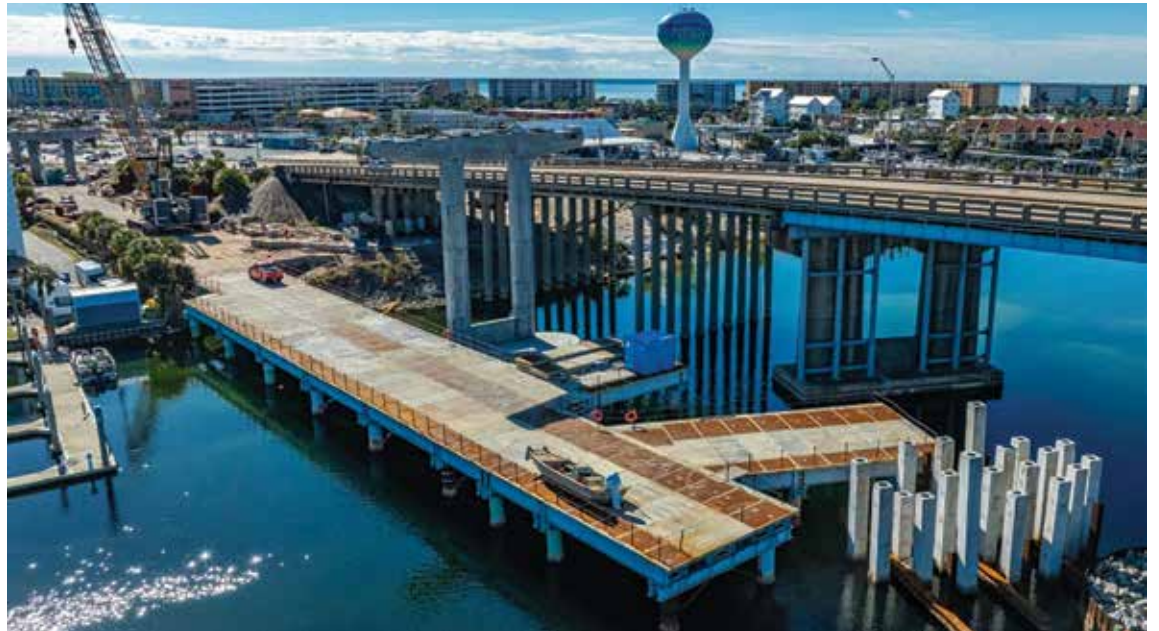
This recent aerial photo (taken north of Brooks Bridge looking toward Okaloosa Island) shows pile driving and pier construction progress in the Santa Rosa Sound. (FDOT)
